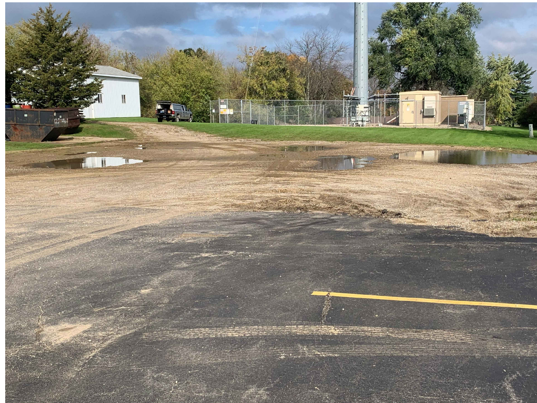
3 C2 EXISTING STORM WATER PROBLEM AREA SCALE: NONE
