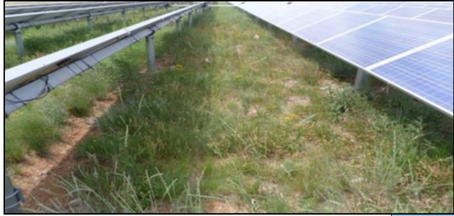
National Renewable Energy Laboratory
