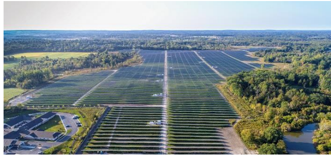
Lapeer Solar Park; DTE Energy
