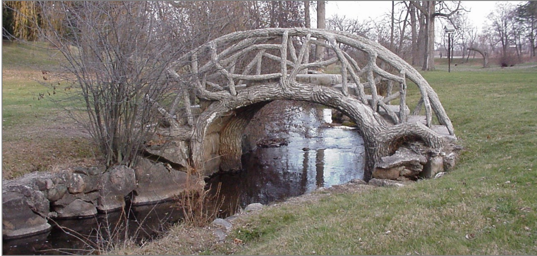
'Trabajo Rustico' Pedestrian Bridge (i.e., 'Rough Work'/Made To Look Like Wood) McCurtie Park | Somerset Township
