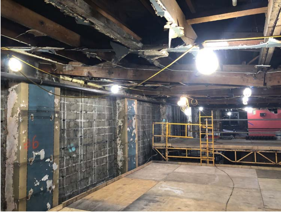
PHOTO #1 – Existing Truss shown extreme sag. Drop is evident on right side.
