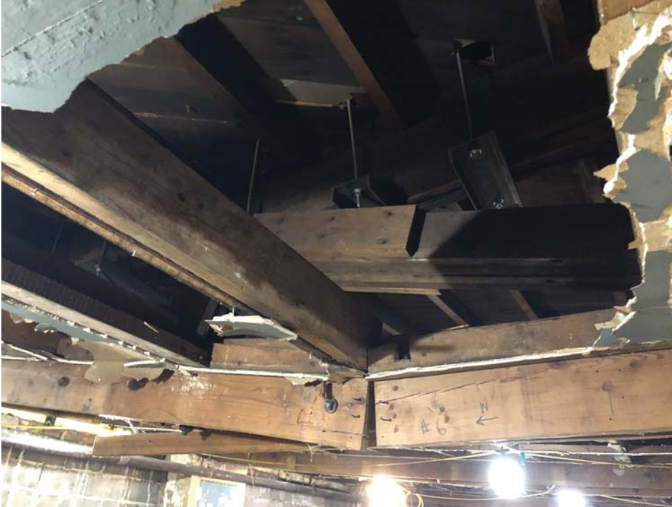
PHOTO #3: Existing top chord repair to be removed to allow for proper roofing to be installed.
