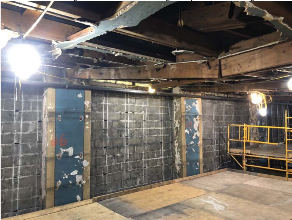
PHOTO #2: Existing Truss shown extreme sag. Drop is evident on right side.
